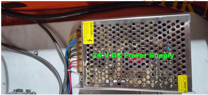
Fig12- Main DC 24V power supply
